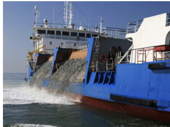
(b) Installation of a stone layer with a side stone dumping vessel (Source: Van Oord)
