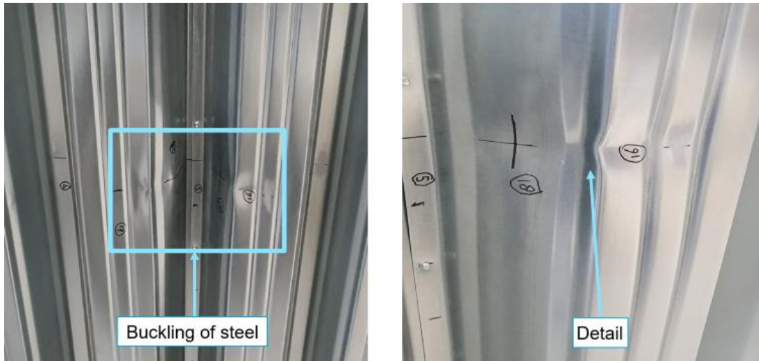
Figure 45 Buckling in the steel at load location.
