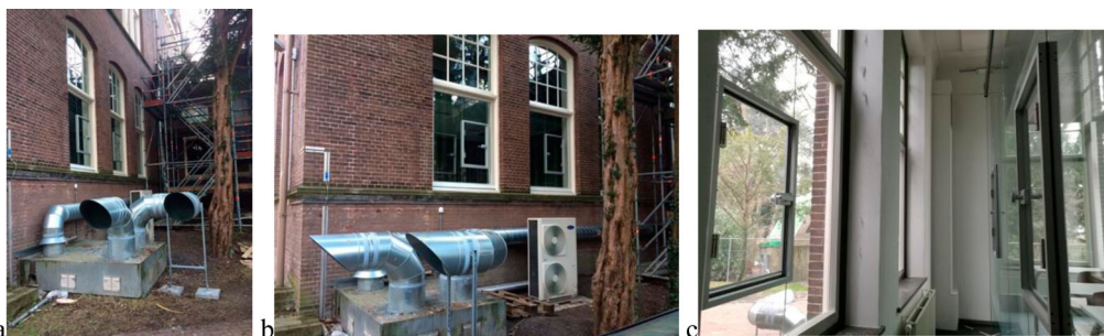
Figure 7. Current situation of the inlet and outlet (a), the cooling system (b) and the 'window-in-window' construction (c).
