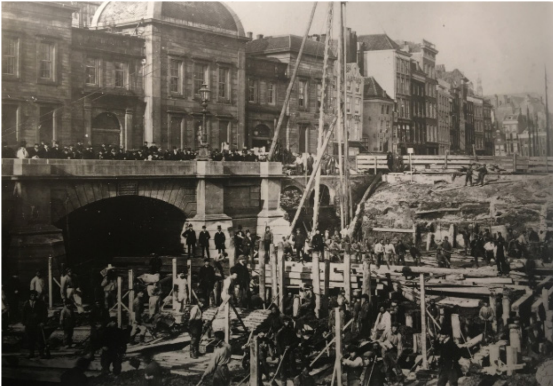
'Pile-driving operations in the damping of the binnenrotte [Inner Rotte] to prepare for the railroad viaduct. Hammer hoisted by means of steam power. In front of the New Exchange Building.' 1875 (Rotterdam City Archives)
