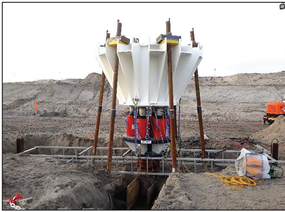
Figure 3. Pile test frame and the reaction anchors used at the Maasvlakte test site
