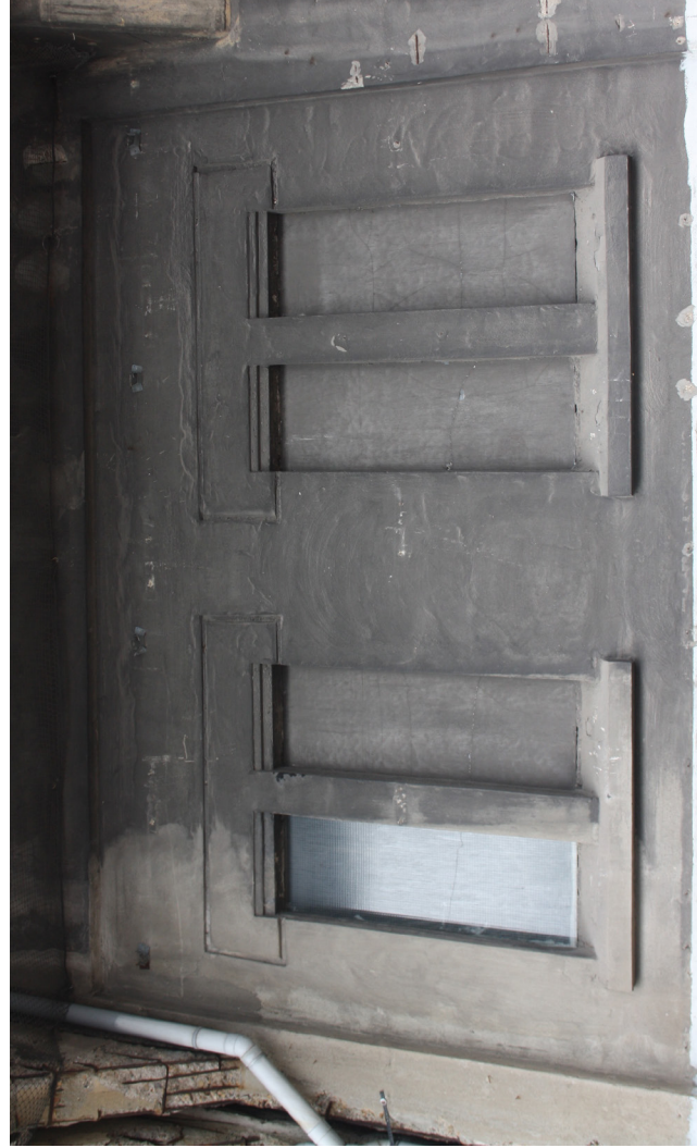
Exterior of the Katoenveem with the lintel detail around the windows. Own image 2016.
