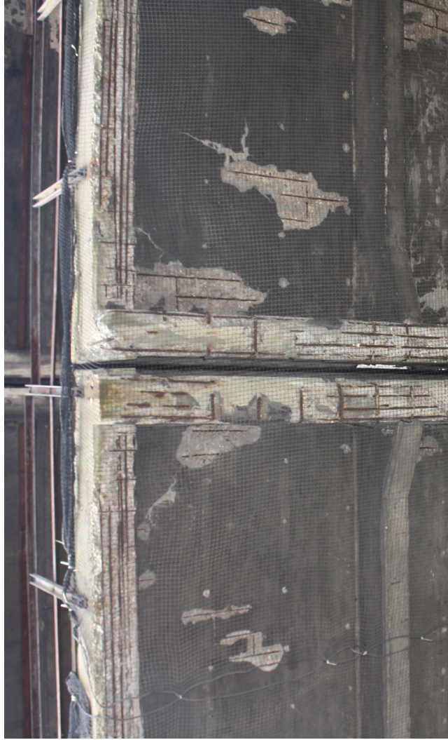
Damage on the exterior of the Katoenveem including the netting put up by the municipality. Own image 2016.
