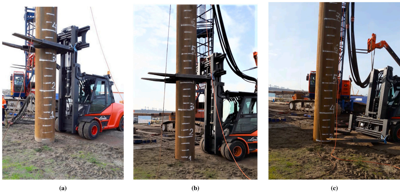
Fig. 9. (a) First, (b) second and (c) third installation phases of an ATP.
