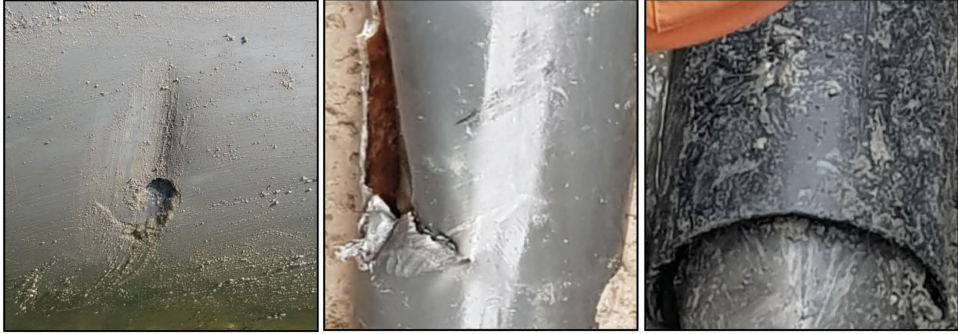
Figure 3.9: In-situ footage after excavation of pipes A-3 (left) and B-2 (middle) with break due to third party impact, and pipe B-3 (right) with crack due to poor installation quality.
