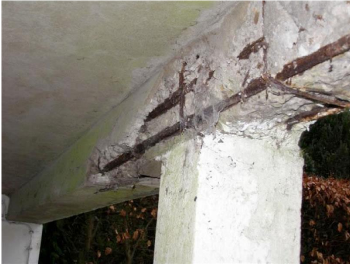
FIGURE 8: CORROSION OF CONSTRUCTION (DE BETON GROEP N.V., 2018)
