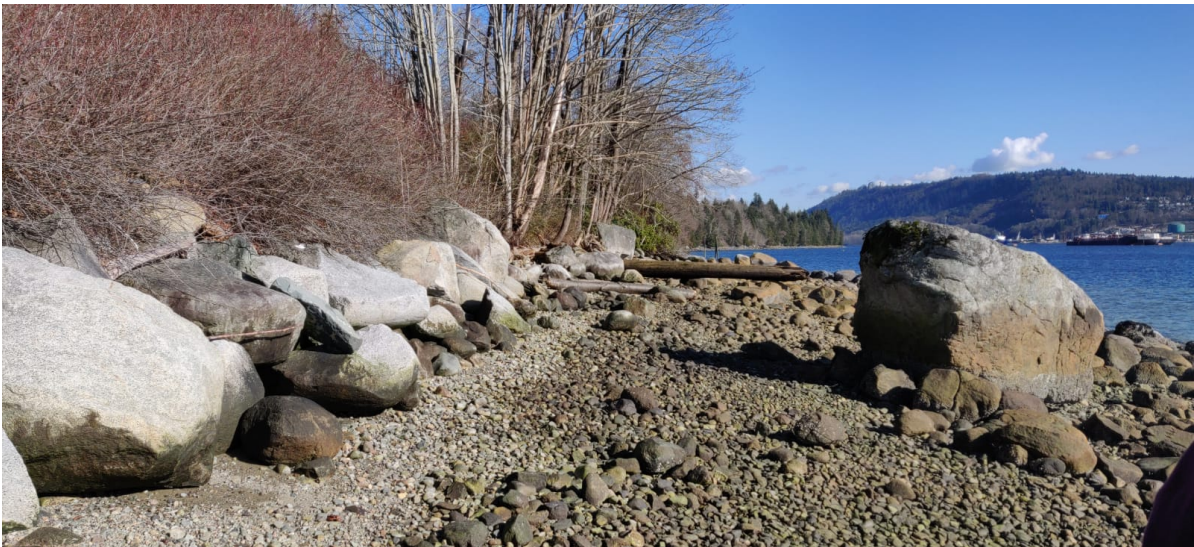
Figure K.3: Site visit project site of the Tsleil-Waututh Nation; picture of previous placed rip-rap with vegetation behind the rip-rap
