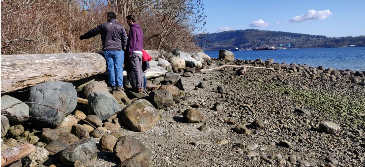
Figure K.5: Site visit project site of the Tsleil-Waututh Nation; Mike showing us the erosion and scarp behind the trees used as extra shoreline protection
