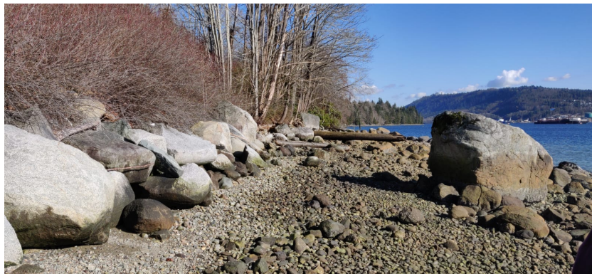
Figure 7.1: A site visit at SWN showed erosion behind the currently placed rip rap
