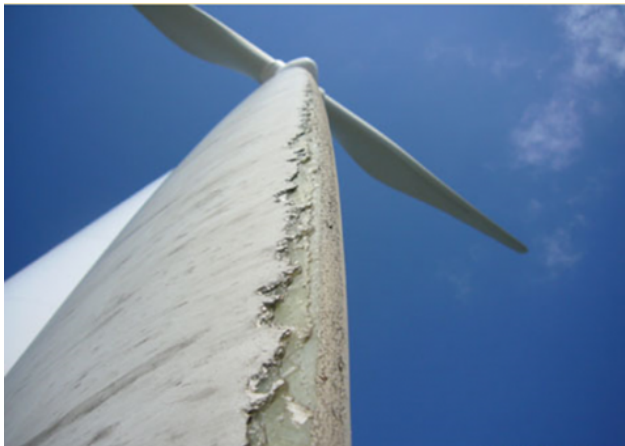
Figure 1.1: Leading-edge erosion damage on a wind turbine blade; photography reproduced from Telene (2021).
