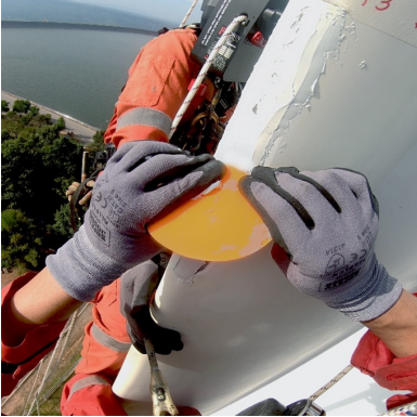
(a) Rope technicians applying a leading-edge repair product; photograph reproduced from Belzona (2022).
