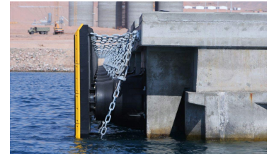
(b) Overview of Super Cone (SPC) fenders on a quay wall [35]
