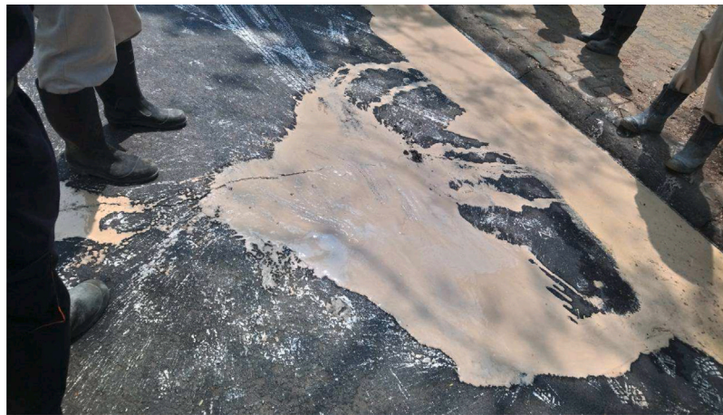
Fig. 8. Blowout case in Hochiminh Metroline No. 1 at the chainage of Km1 + 154.4.
