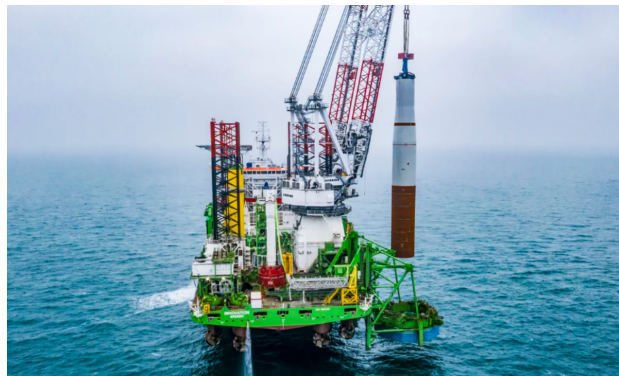
(b) A fully jacked-up installation ship. The monopile is seen just before it gets lowered into the fixed pile gripper frame
