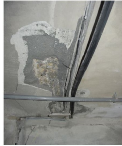
(b) Concrete cracking at dilation joint(Leeuw, 2008)
