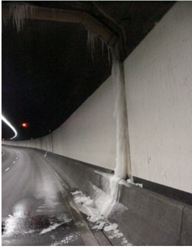
(a) Joint leakage(Leeuw, 2008)
