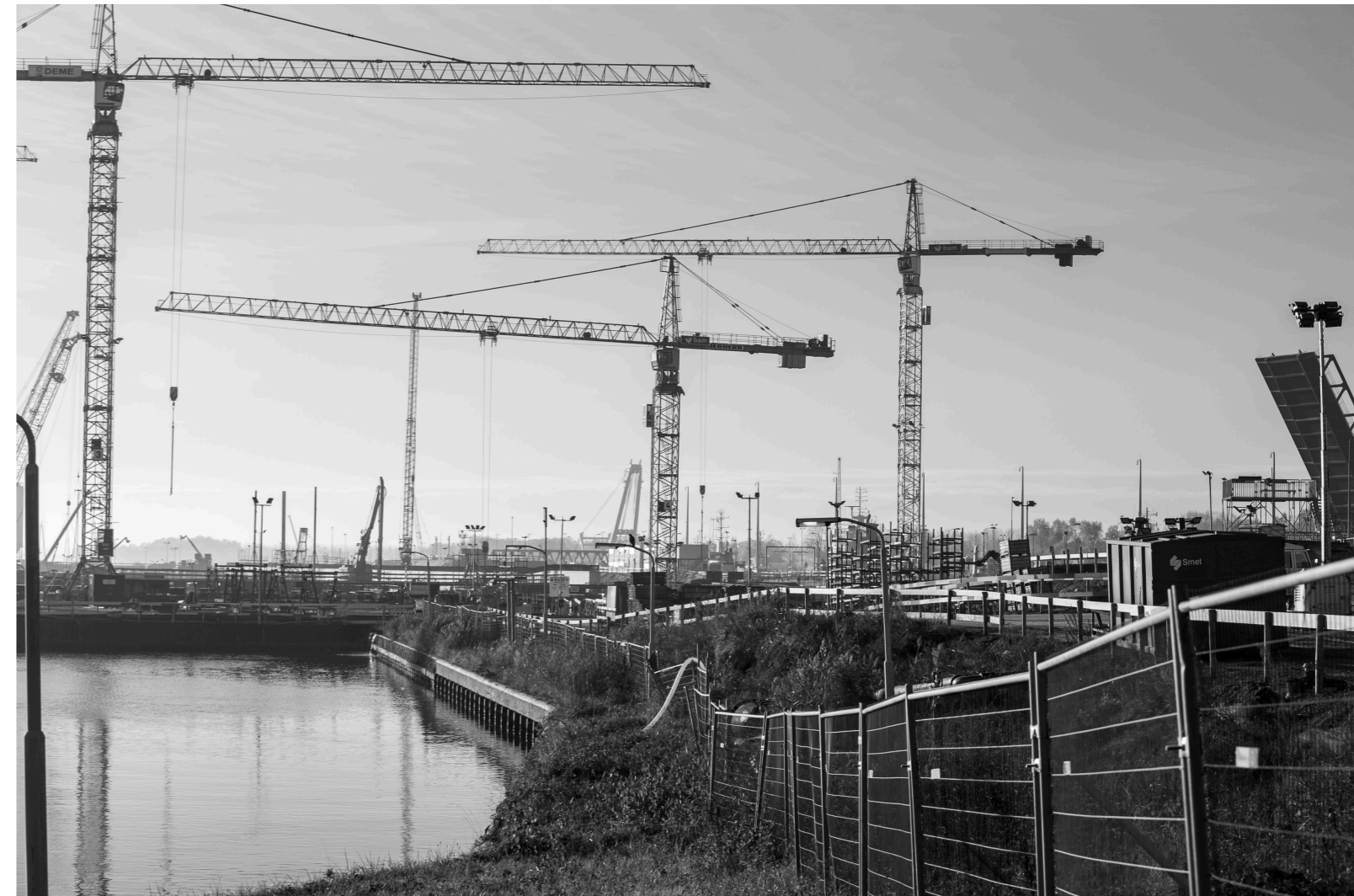
5.14 Current focus on expansion of ports and becoming a global hub: sluice extension in Terneuzen as part of The North Sea Port developments
