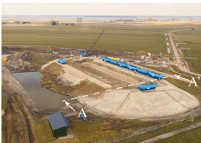
Fig. 7. Aerial photo of the Eemdijk ring-shaped test dike, with slope instability of the conventional (ground) dike (left). The test dike with sheet pile, is located on the right side. Image courtesy of Eric Feijten/NOS (Feijten, 2018).
