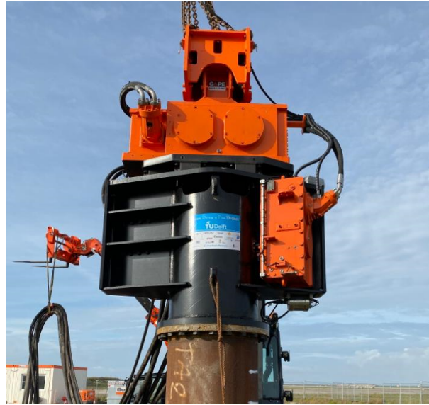
Figure 1: The GDP shaker connected to a pile via a bolted flange connection.
