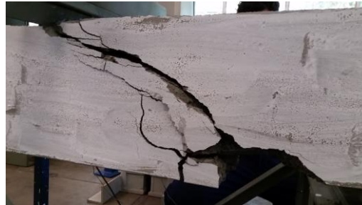
Figure 1.9 – Transverse shear failure of a reinforced concrete beam[33]
