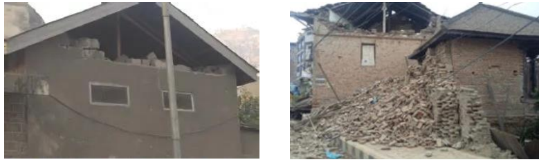
Figure 2.14: Out of plane collapse and overturning of gable masonry [46, 56]
