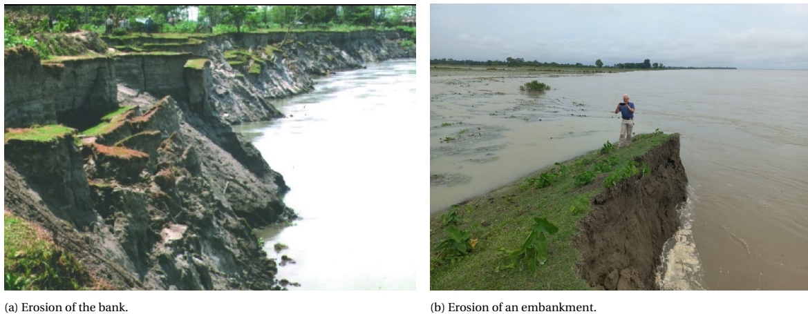
Figure 2.5: Bank erosion along the Brahmaputra. Left image from Sarkar (2017) . Right image courtesy of Sanjay Giri.
