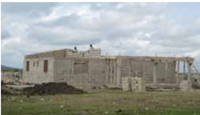
Figure 32 Illegal construction on the Site (Forestry Commission, 2018)
