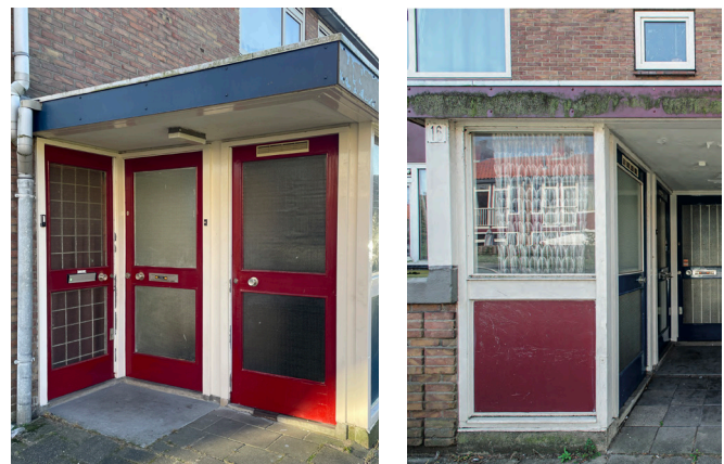
Figure 4.43: Detached entrance portal of the duplex typology in the Louis Couperus neighborhood (by author).
