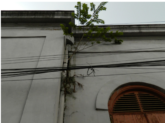
Gutter and Biological Growth
