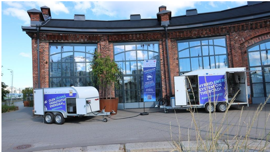
Figure 1. Mobile hybrid energy system built in two trailers. The left trailer includes energy storage system, and the right one encloses power electronics system and high power charging station for electric vehicles. Technically versatile system offers excellent open innovation ecosystem for modern electric drives of smart energy transition. [3]
