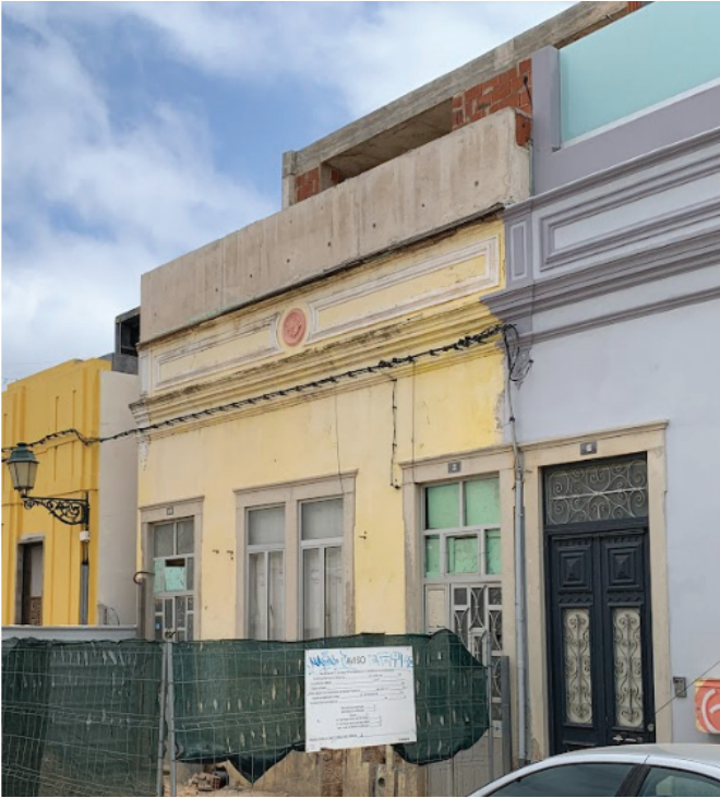
Figure R6. Building in Sao Francisco where another level is being added
