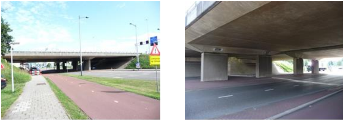
Figure 1 Side view (left) of investigated bridge and columns supporting the decks (right)
