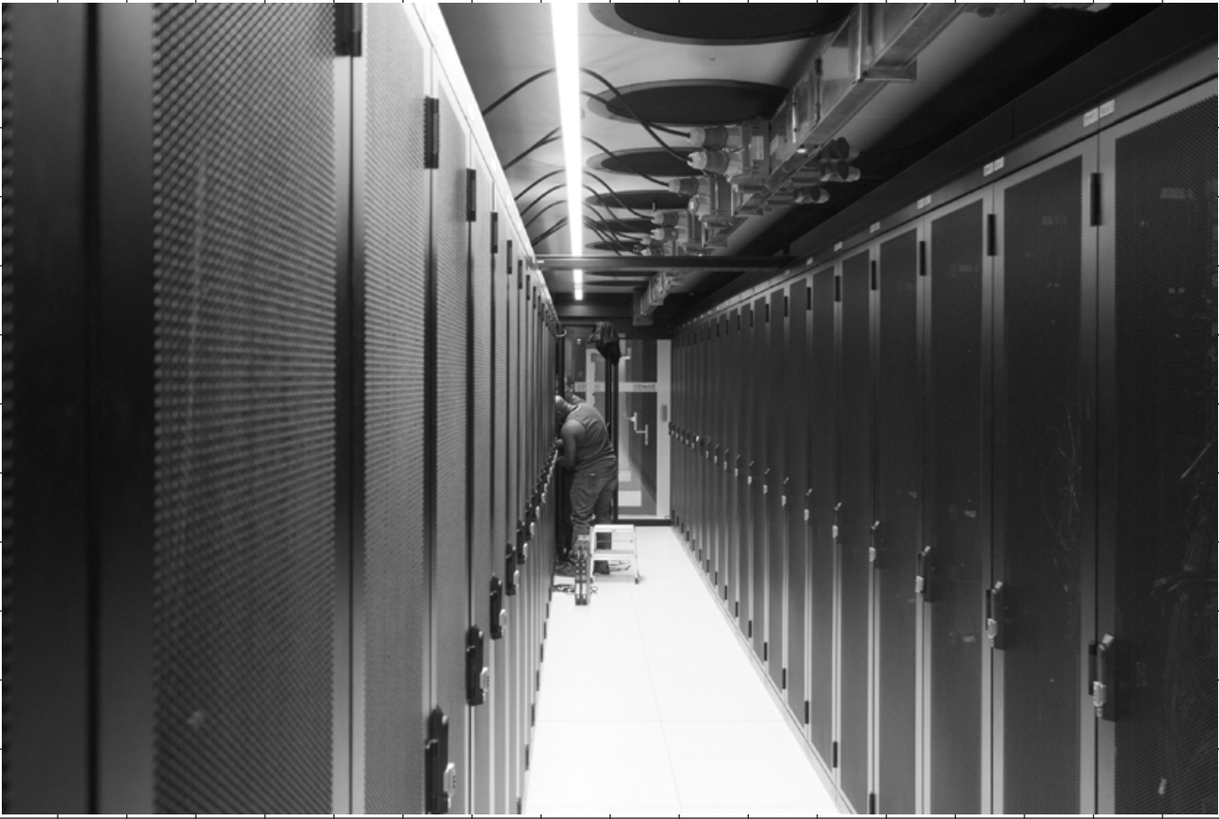
Data Centre SmartDC, Rotterdam. Photo by Johannes Schwartz
