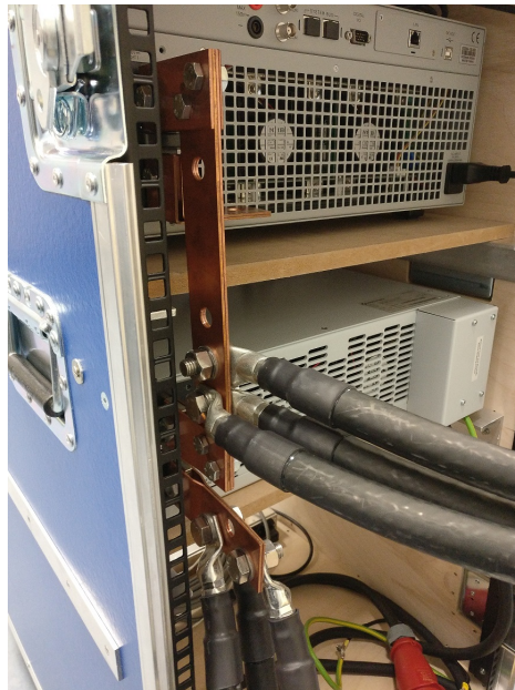
Figure 4.18: Additional copper bus bar for cable connections
