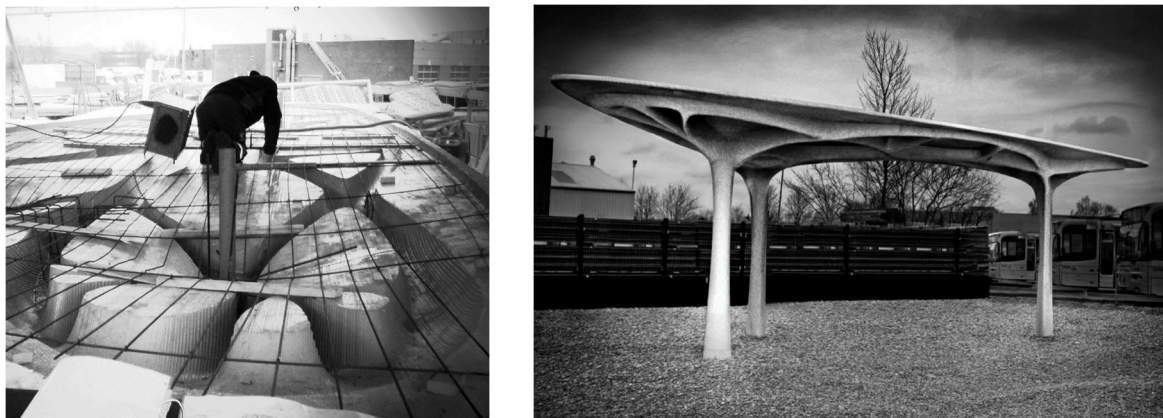
Figure 2-3: The Unikabeton Prototype. a) Assembly of polystyrene moulds at the building site. b) Finished structure [17].
