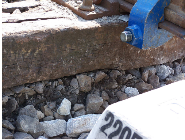
Figure 1.2: Severely worn ballast stones under an old sleeper. Compared with the new ballast stones nearby with sharp edges, the worn ballast stones have become rounded in shape and covered by dust. This problem is called the "foul" of the ballast, meaning that the ballast stones have been crushed, provide less drainage, move less, and have less elasticity, leading to a reduction in their friction dissipation.
