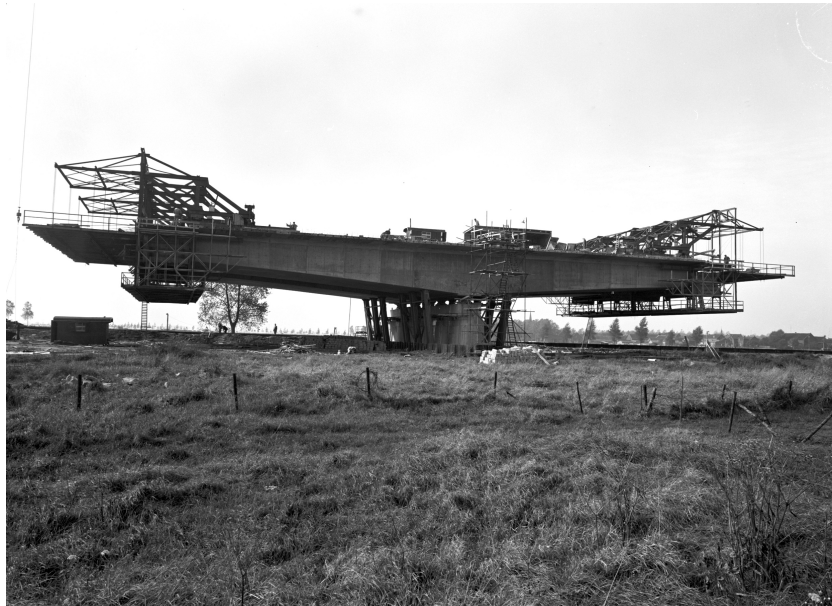
Figure 1.1: Construction of the Maasbrug near Wessem, the first balanced cantilever concrete bridge in the Netherlands [11].
