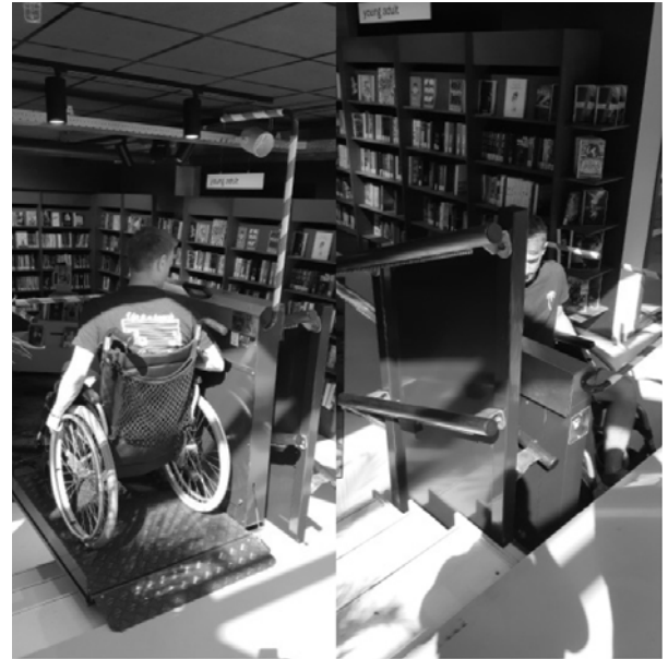
Fig. 2.12 (by author): Wheelchair lifts in public buildings (Delft library) ( aid )
