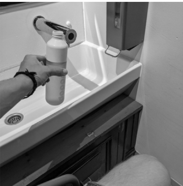
Fig. 2.11 (by author): Awkward taps in public buildings ( barrier )
