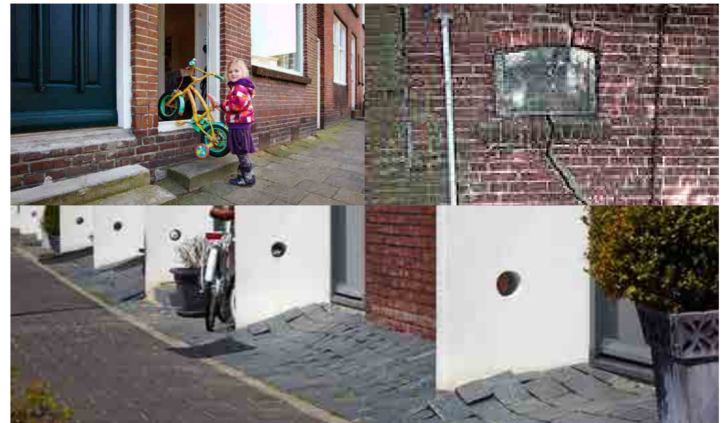
Figure 2.3: Damages because of subsidence. Source: http://www.slappobodem.nl/
