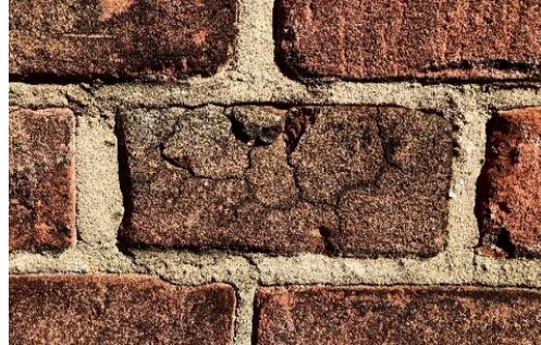
Figure 3-6 localized damage in brick
