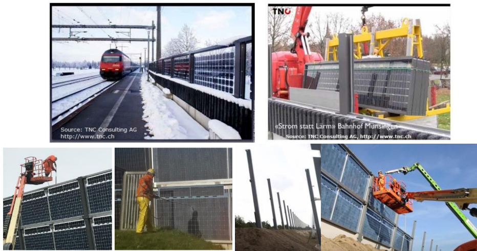
Figure 5 - 4: Compilation of PVNB photos (top row) Swiss cassette type photovoltaic noise barrier in operation and during installation (bottom row) Solar Highways Dutch experimental photovoltaic noise barrier (~240kW) during construction, installation and maintenance periods
