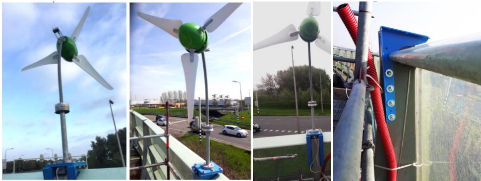
Figure 5 - 3: Photos during construction of the highway experimental set-up of highway micro wind turbine noise barrier highlighting the structural integration features such as the blue flange
