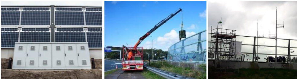
Figure 5 - 5: Photos of (left) Grid interconnection of the Solar Highways PVNB 240kW demonstration in the Netherlands – Copyright of Heijmans, (middle) installation of electric cast for interconnection to low voltage network for the MWTNB experiment (right) installation of the micro wind turbine on the noise barrier
