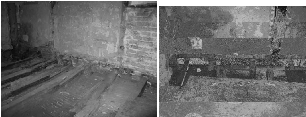
Figures 9 and 10: Rotten structure and typical steel reinforcement.
