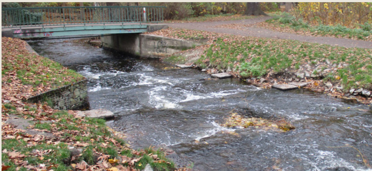
Figure 1.6. Fish ladder in the Panke River in Schlosspark Niederschönhausen (Geißler, n.d.)
