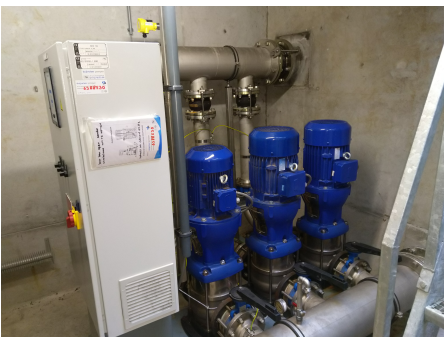
Figure F.5: Pump at inlet
