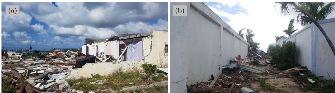
Figure 4.14 Damages observed in Sint Maarten due to Hurricane Irma. (a) Simpson Bay. (b) Billy Folly.
