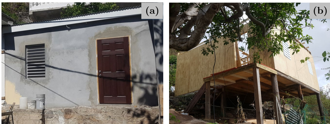
Figure 2.17. Observed reconstruction in the island. (a) With stronger materials (block, concrete). (b) With weak materials (wood).
