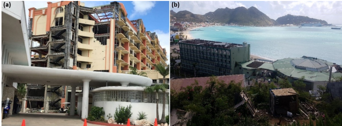
Figure 2.18. Damage to hotel infrastructure. (a) Sonesta Maho (Simpson Bay) (b) Great Bay Hotel (Philipsburg)
