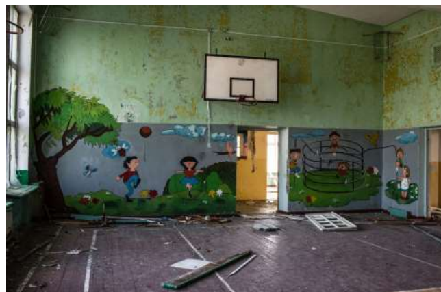
Figure 29: Abandoned school building in Vorkuta (Demyanenko 2020)
