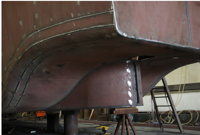
Figure 3.11: Example of a pram-shaped stern, including a skeg (photo by René Rapati, Groenendijk & Soetermeer).
