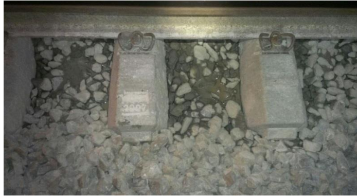
Fig. 1. Hanging sleepers and track degradation (mud pumping)
