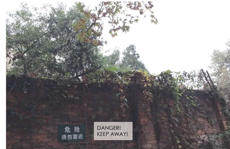
Aging dangerous wall.
