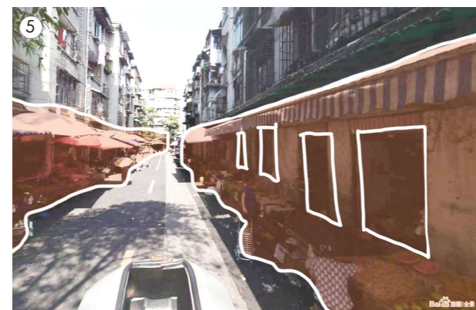
The first floor housing on both sides of Neighborhood Street have been converted into shops by breaking down the walls.
