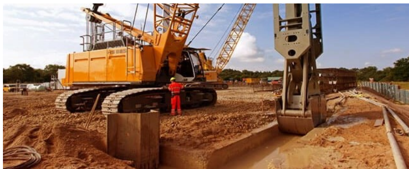
Figure 2.17: Crane excavating a trench during construction of a diaphragm wall. Photo by GKV Infrastructure Piling Contractors.
