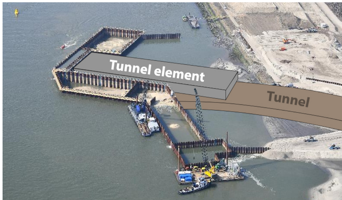
Figure 3.5: Construction of the cofferdams on the North side with the tunnel placement indicated. Adapted from BAAK.
