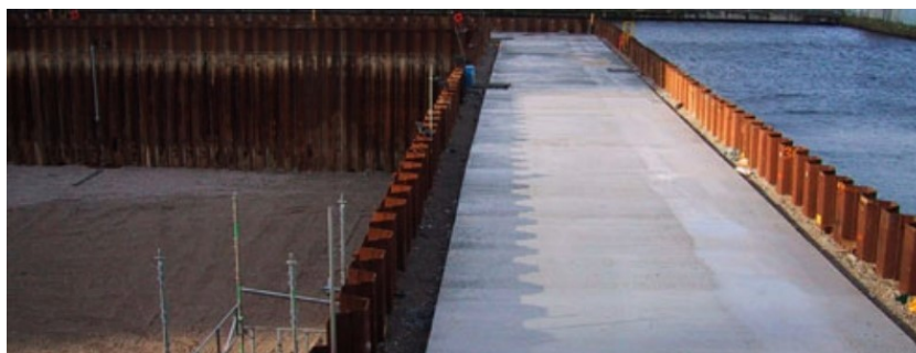
Figure 2.19: A cofferdam with a concrete slab on top. Photo by Dawson Wam.
