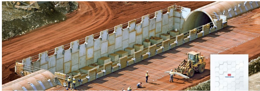
Figure 2.21: The application of a 'terre armee' method to construct a deep excavation. Photo by Noise.
