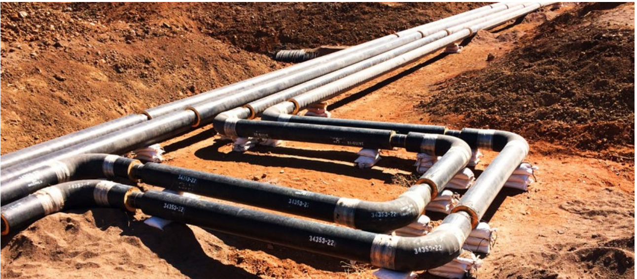
Figure 1: An example of an expansion loop (photo credit: VHM Solutions Pty LTD)
