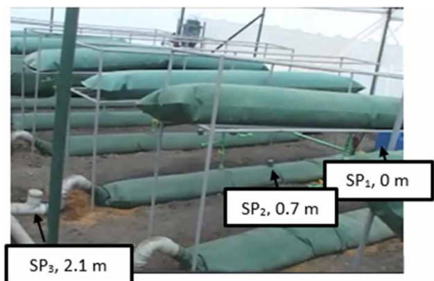
Figure 1 | Plug flow digester layout; reactors on the floor, biogas collection bags directly above; sampling points are indicated (SP 1 , 2 and 3).
