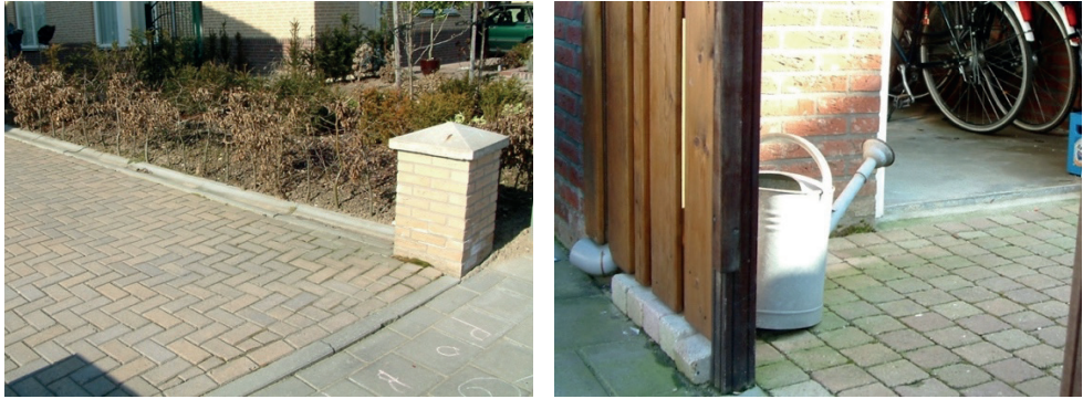
Figure 4-1. Two cases (#13 and #15) of technical failures in SUDS with a failing function of conveyance. Left: an obstacle interferes with the transport of water by an open gutter. Right: due to insufficient slope of the garden, the storm water flows into the shed.
