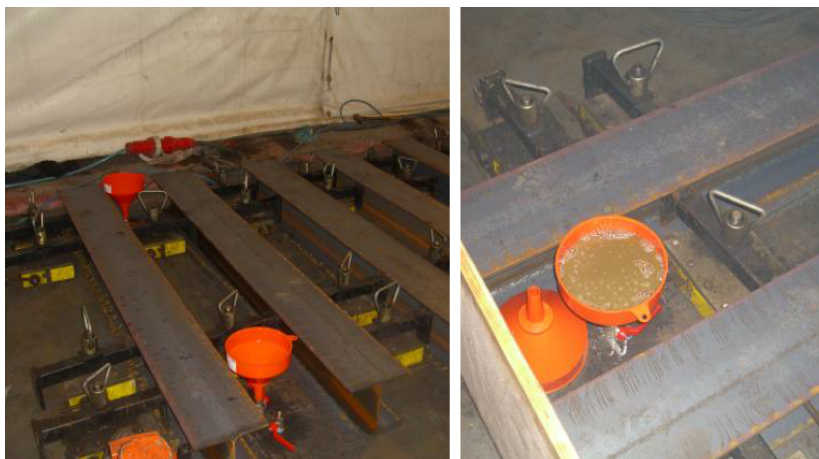
Figure B-3: (a) Restraint beams are added to keep the top faceplate in place during pressurized injection. (b) Pre-drilled holes in the top faceplate enable the polyurethane from escaping the cavity when entirely filled. [Source: SPS - Engineering Details, Intelligent Engineering Limited]
