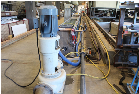
(a) Pump one, used to regulate the discharge
